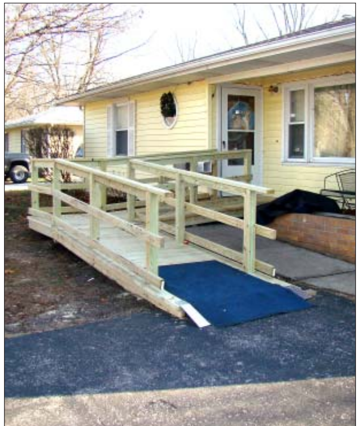
One of our ramp projects which was completed near the end of 2011.
